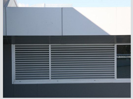
MAL 100mm Single Bank - Napier St, GHD Building, Auckland.
