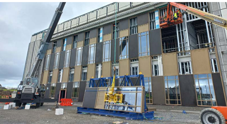
Latter Day Saints, Auckland site installation - PW1000 unitised curtainwall with integrated glazing, aluminium louvre and non-vision panel.
