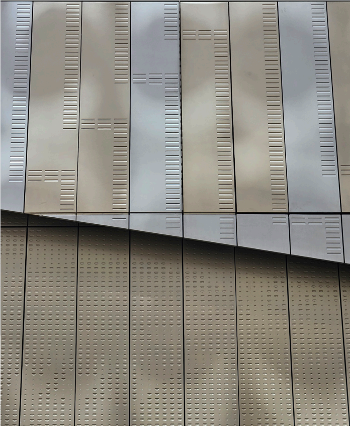
Detail of the prefabricated unitted embossed aluminium panels installed on the National Archives building in Wellington.
