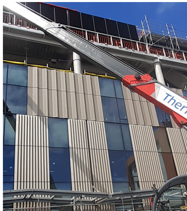
Taranaki Base Hospital Extension - under construction with High Performance PW100 unitised curtainwall integrated with Thermoplank unitised rainscreen.
