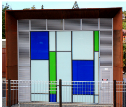
Door with MAL 40mm Single Bank & curtain wall with integrated MAL 100mm Single Bank - Vector Substation, Auckland.
